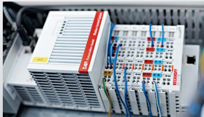
The condition monitoring system is supplied ready for operation, installed in a compact terminal box.
