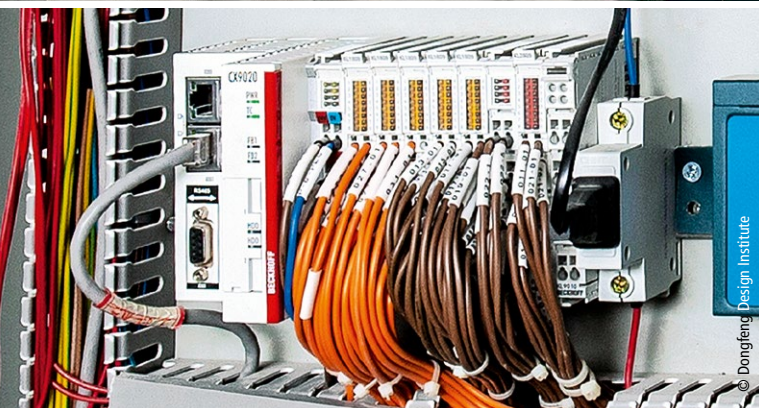
CX9020 Embedded PC with directly attached Bus Terminals in a building control cabinet
