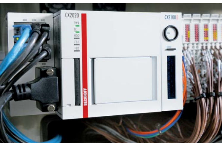
A CX2020 Embedded PC with a directly linked I/O terminals and TwinCAT 3 automation software is used as the central controller for the M1 synthesizer.
