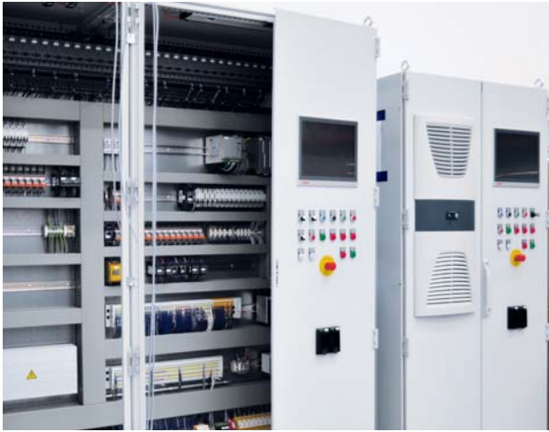
Both the tower control cabinet (right) and the nacelle control cabinet (left) of the turbine prototype use a CP2915 multi-touch Control Panel with a 15-inch screen for easy operation.
