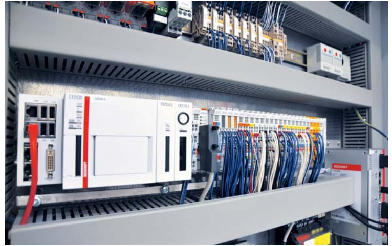
The Beckhoff CX2030 Embedded PC (left) in the tower control cabinet controls the entire system, while the C6930 control cabinet IPC (right) handles visualization, monitoring and remote access in the prototype installation.
