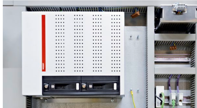
A C6650 control cabinet Industrial PC with multi-core processor is used for higher-level control and monitoring of the entire Lisocore® production plant.
