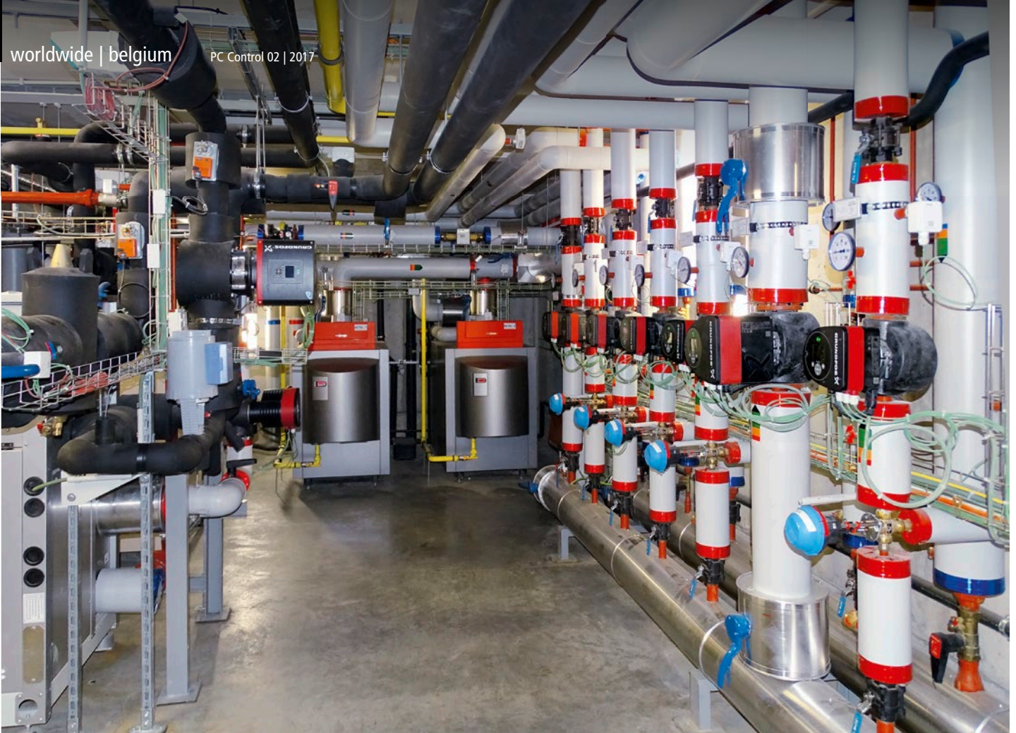
The HVAC control of the university building encompasses over 4,000 I/O points.
