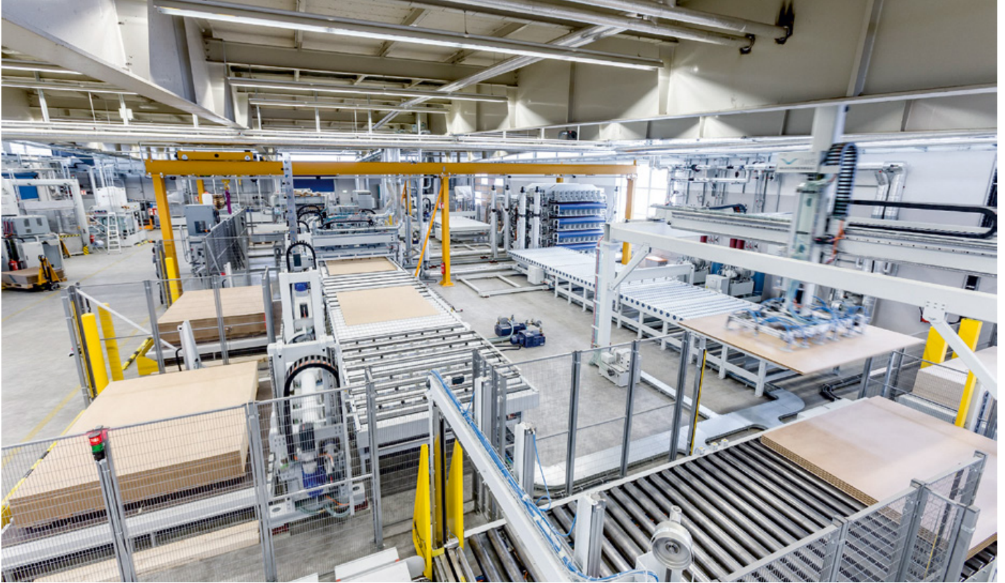
The rectilinear arrangement of the processing stations results in a highly compact and powerful machine installation.
