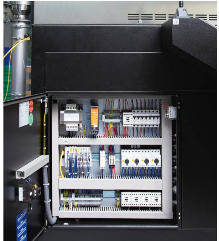
The I/O system is controlled via EtherCAT.
