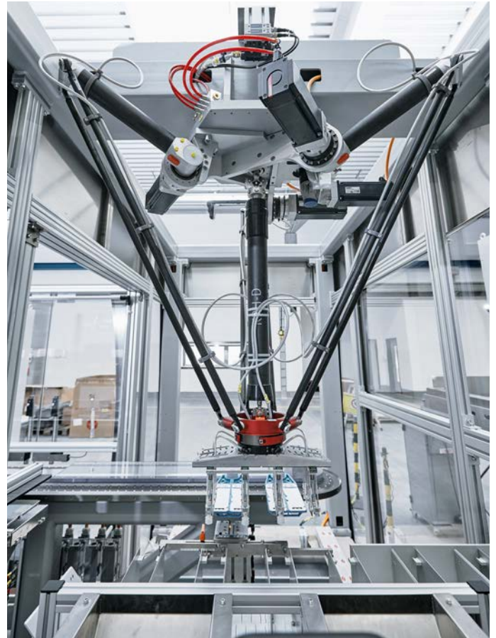
The two HSPP systems at the start and end of the labeling and grouping unit employ dynamic Beckhoff drive technology and are controlled together with the XTS via a single C6930 control cabinet PC.
