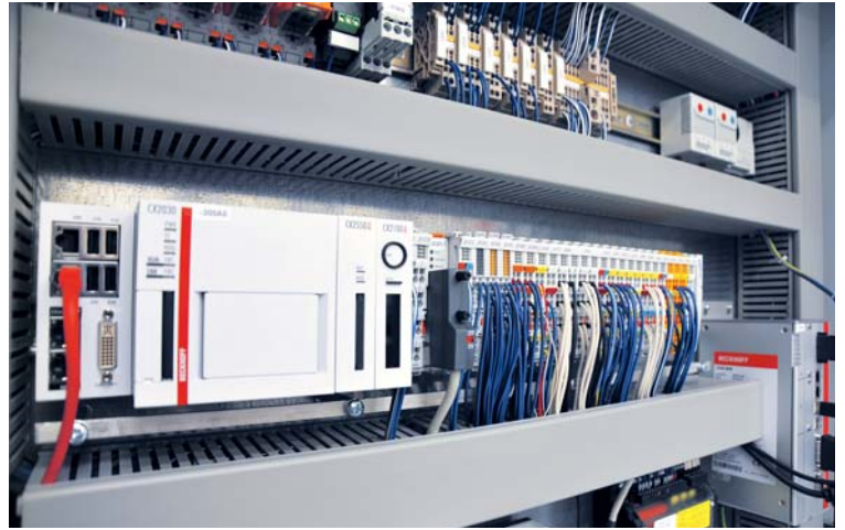
The Beckhoff CX2030 Embedded PC (left) in the tower control cabinet controls the entire system, while the Beckhoff C6930 control cabinet IPC (right) handles visualization, monitoring and remote access in the prototype installation.
