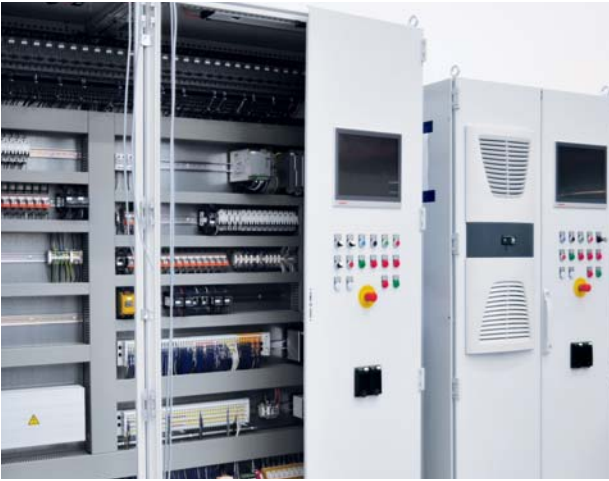
Both the tower control cabinet (right) and the nacelle control cabinet (left) of the turbine prototype use a Beckhoff CP2915 multi-touch Control Panel with a 15-inch screen for easy operation.
