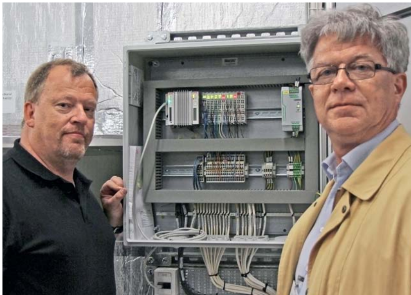
Widex Project Manager Allan Ebert Skotte (left), responsible for all technical building installations, and Claus Clausen, Managing Director of Beckhoff Denmark
