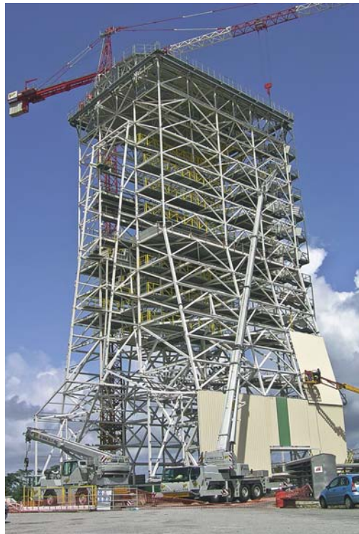
The Soyuz mobile gantry at the spaceport in French Guiana under construction. The mobile gantry is 52 meters (171-ft) high and can approach the already built rocket on rails. The payload is installed in the nose of the rocket from the mobile gantry at a height of 36 meters (118-ft).
