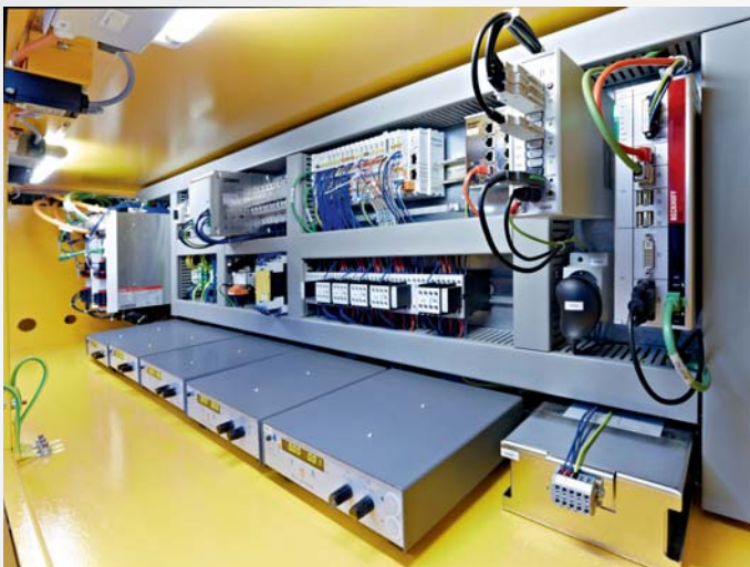
Each of the 91 undulator cells is controlled via PC-based control. The system features a C6925 control cabinet PC (right), numerous EtherCAT Terminals (center), and two AX5206 Servo Drives (left).
