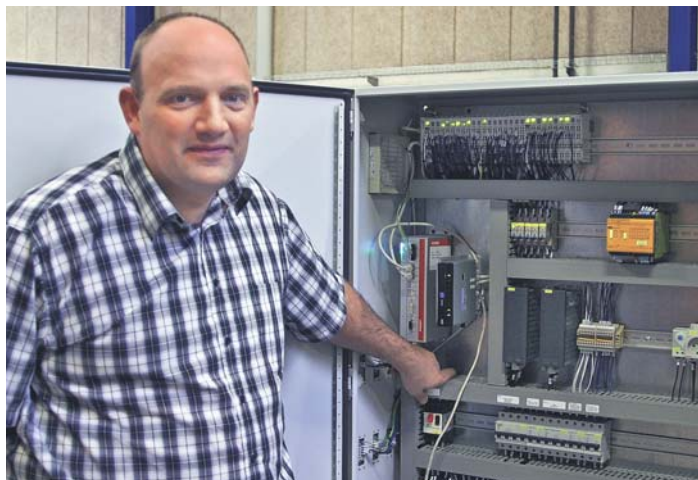
Morten Pipper, Managing Director of Obel-P Automation A/S, at the control cabinet of the pressing line
