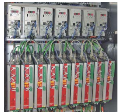
25 electric motor-driven servo axes and 12 hydraulic servo axes are controlled by Beckhoff AX2003 Servo Drive systems.
