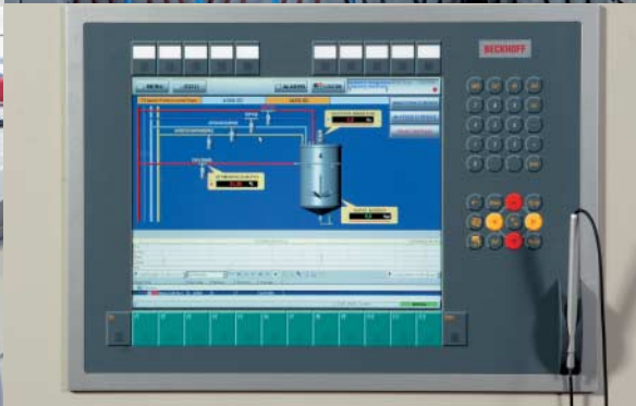
Control Panel running the SCADA software with SQL process monitor.
