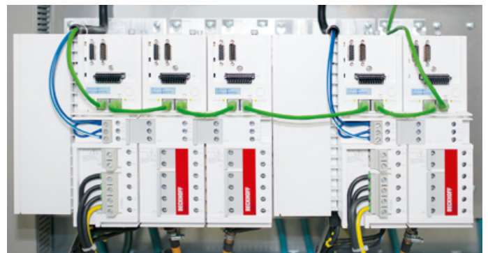
The control system for the whole line handles more than 2,500 data points. The hardware includes 73 AX5000 Servo Drives (shown here), 51 EtherCAT Couplers, 778 EtherCAT Terminals, and 22 EtherCAT Box I/O modules.
