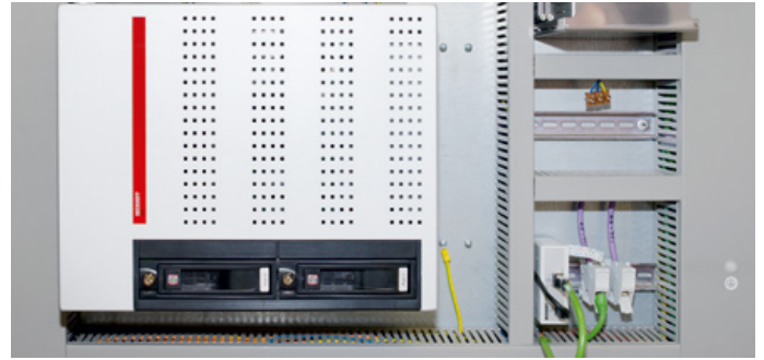
A C6650 control cabinet IPC with multi-core processor technology controls and monitors the entire production system for Iisocore® composite panels.
