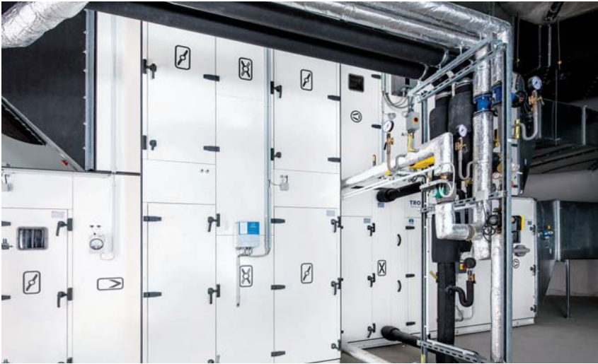
Nine X-Cubes, configured as air supply and extraction units with highly efficient cross-flow plate heat exchangers, ensure perfect conditions in the Buchholz Galerie at all times.
