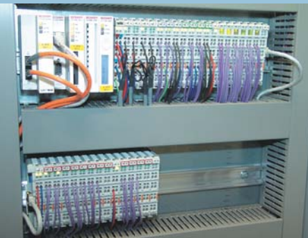
Control cabinet of the gearbox test rig for the tail rotor with the CX1000 Embedded PC
