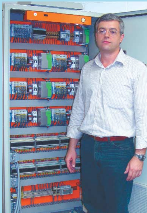
Mauro Poltronieri – director for automation systems at Wheaton Brasil – next to the control desk for the new control system.
