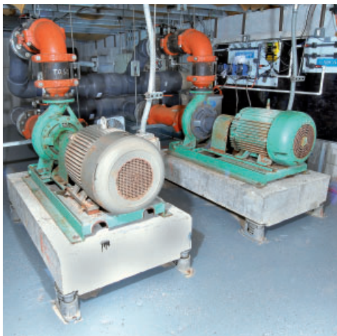
Considering the typical ROI system savings on a single pump running at 60 Hz, the yearly ROI achieved at Toscana North is significant.
