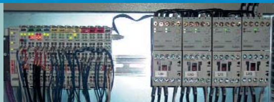
The tobacco cutting line uses more than 400 Power Terminals.
