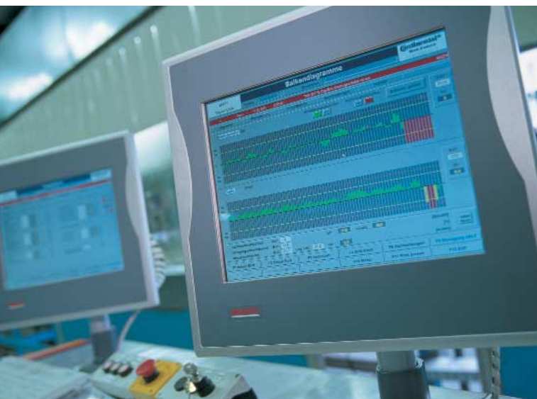
Systems visualization at the control station
